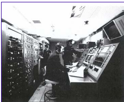
Fig. 13. Cloudcroft control room circa 1974.
